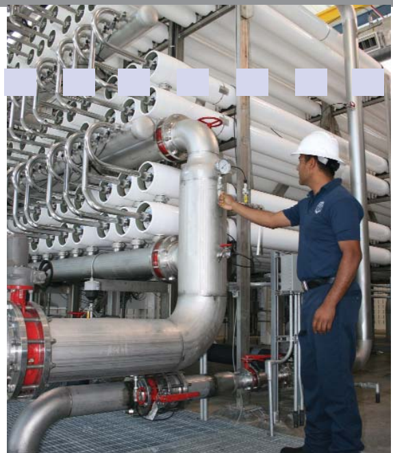
The new desalination plant gives El Paso an additional source of water.
