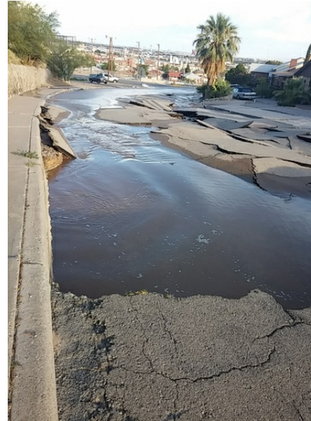
An Aug. 6 water main break destroyed portions of Ingersoll Way and Alabama Street.
