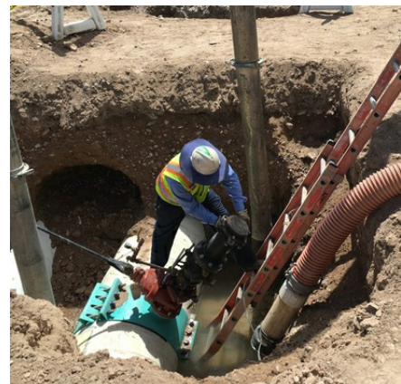
A contractor's worker taps into the 42-inch Frontera Force Main to replace one of nine failed valves.
