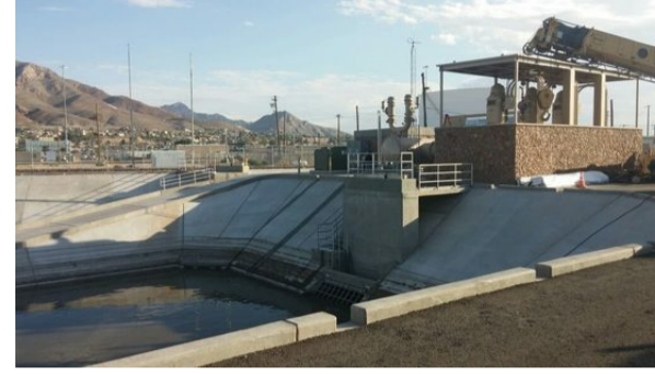
Magnolia Pump Station
