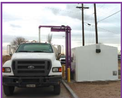
Reclaimed water dispensing station.
