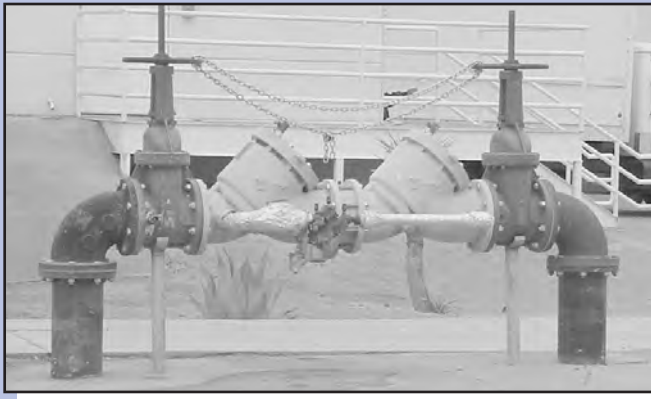
Sample of a large backflow unit.
